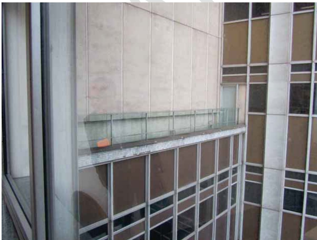
ALUMINIUM WINDOW FRAMES, GOLD SPANDRELS, A STRIP OF THE ORIGINAL MOSAIC TILING AND THE C1972 CLADDING WHICH REPLACED THE TILING.
