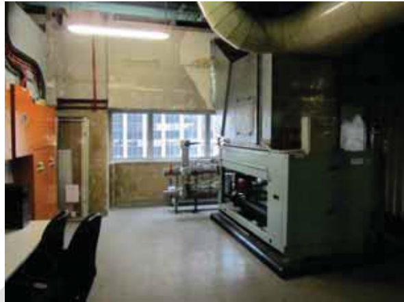
GENERAL PLANT VIEW
