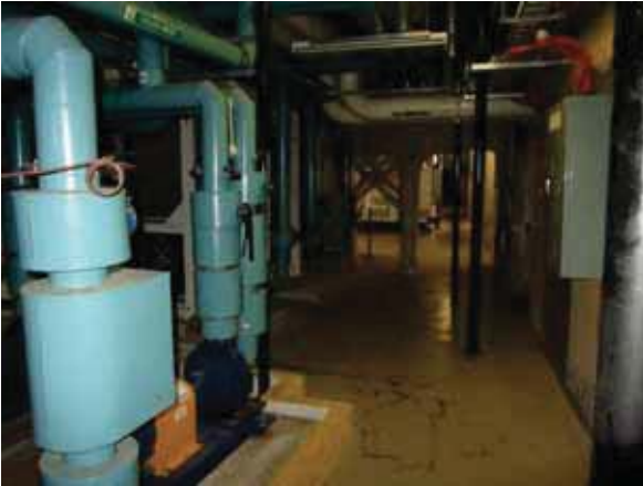
MAINS SECONDARY WATER SUPPLY PLANT
