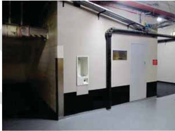
ORIGINAL WATER FOUNTAIN ADJACENT TO THE LIFT CORE (CAR WASH AT LEFT)
