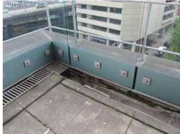
MODERN GLASS BALUSTRADE, DEGRADED CONCRETE DRAINAGE
