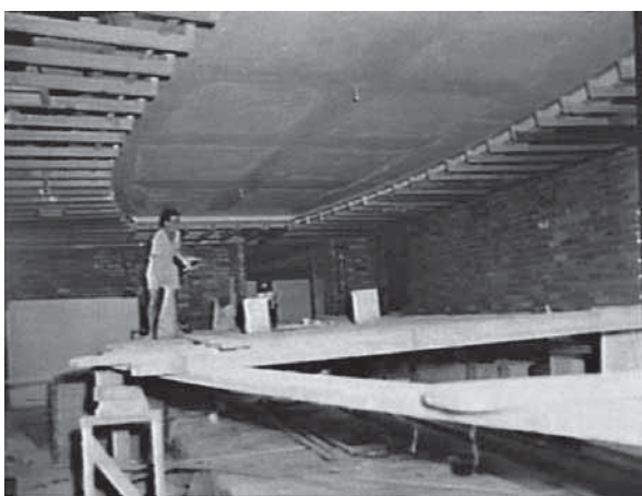
THE BOARDROOM UNDER CONSTRUCTION SOURCE: STATE LIBRARY OF NSW / AUSTRALIAN PHOTOGRAPHIC AGENCY - 11553 - NOV 1961
